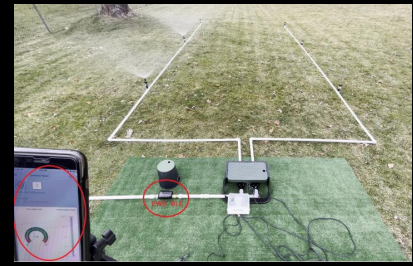
Sprinkler head shutoff
